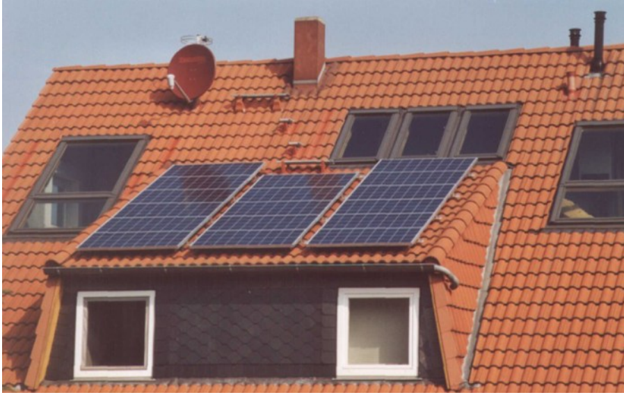
Figure 3.1 This rooftop photovoltaic installation is considered in this example.
